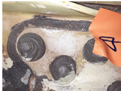
Figure 1 - Pitting corrosion found under microbial growth on a tank surface
